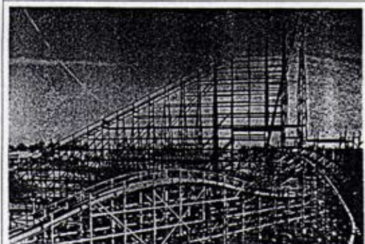
The highest beam is placed 100 feet above the ground on the giant wooden roller coaster structure currently under construction at Worlds of Fun. From this point the coaster train will plummet its passengers 95 feet towards the earth at 53 mph. The new coaster features a combination of thrilling elements including sharp-banking turns intertwined in the giant wooden structure. The $3 million dollar ride, one of the park's largest expansions ever, is scheduled to open on April 1, 1989 when the park begins its 17th season.
