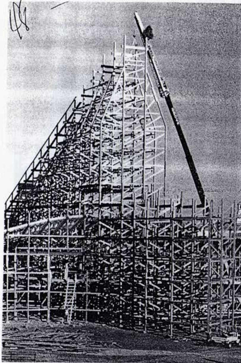
The highest bent is placed 100 feet above the ground on the giant wooden roller coaster under construction at Worlds of Fun.
