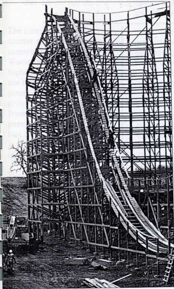
Final work on the 95-foot drop of the Timber Wolf , the new woodie at Worlds of Fun.
